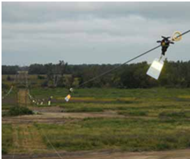
Figure 7.7. Markers on wires can reduce bird collisions by up to 90% (source: Altalink).
