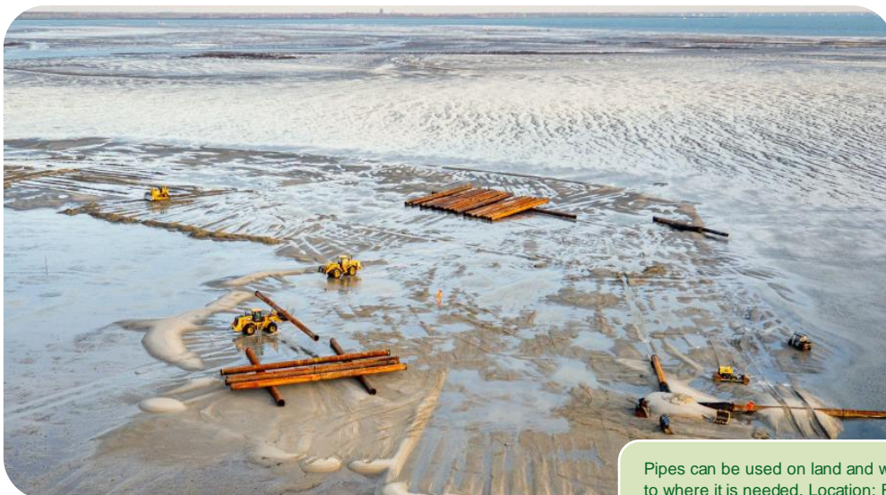
Moving large quantities of sediment requires heavy machinery and skilled labour. Here, sediment is transported on a boat and is pumped through a pipeline to the target area. Location: Roggenplaat island, Oosterschelde, The Netherlands. [Credit: Edwin Paree].
