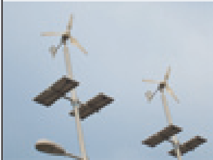
Wind and Solar power Street lights in Kampala
