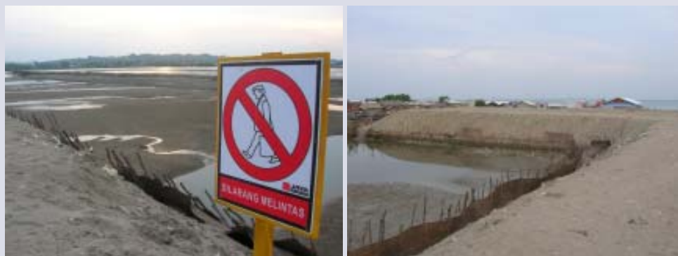
Figure 72. Almost completed embankment sea defence on mudflats at Desa Kedeu Aceh village -Lhokseumawe
